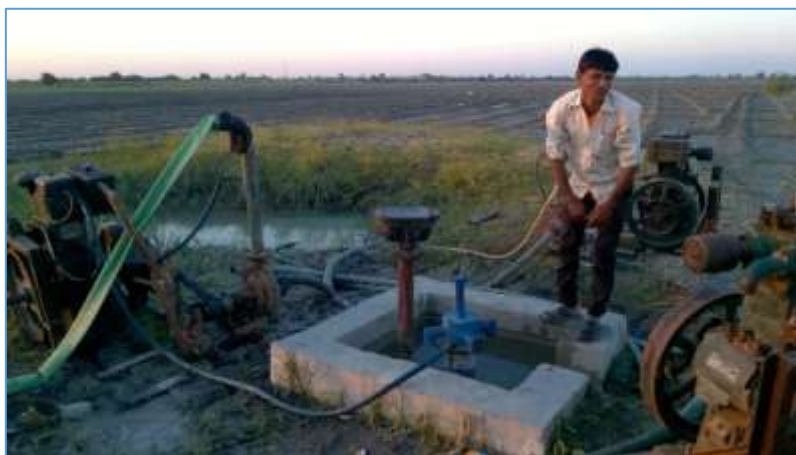
Figure 5. Exit point well as spot for individual pumping, west part SSP, 2015 Source: Photo by Peter Mollinga
